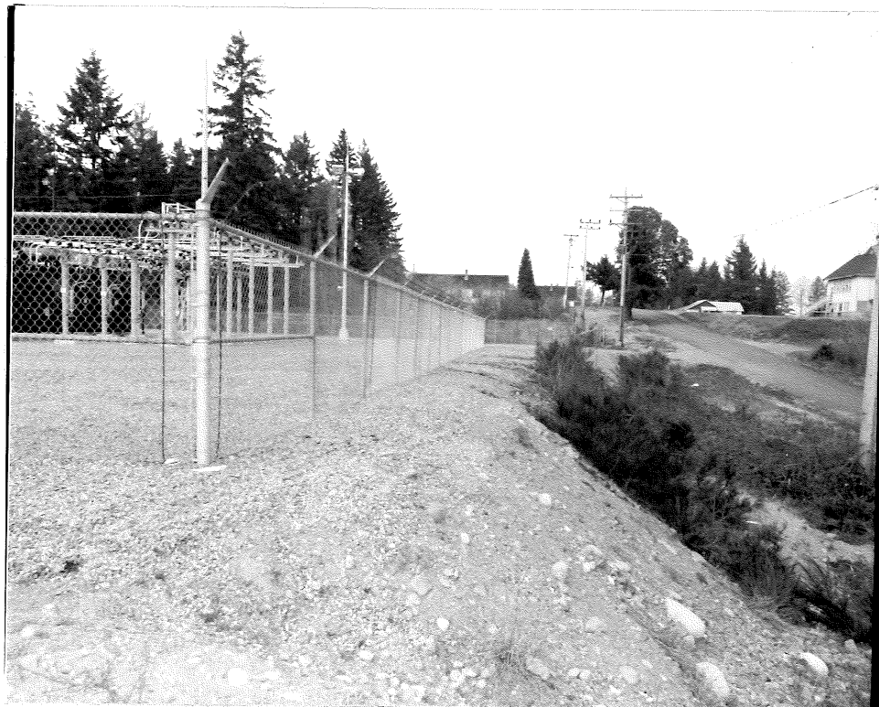
Steep Gravel Bank Showing Erosion and Slow Plant Colonization.
