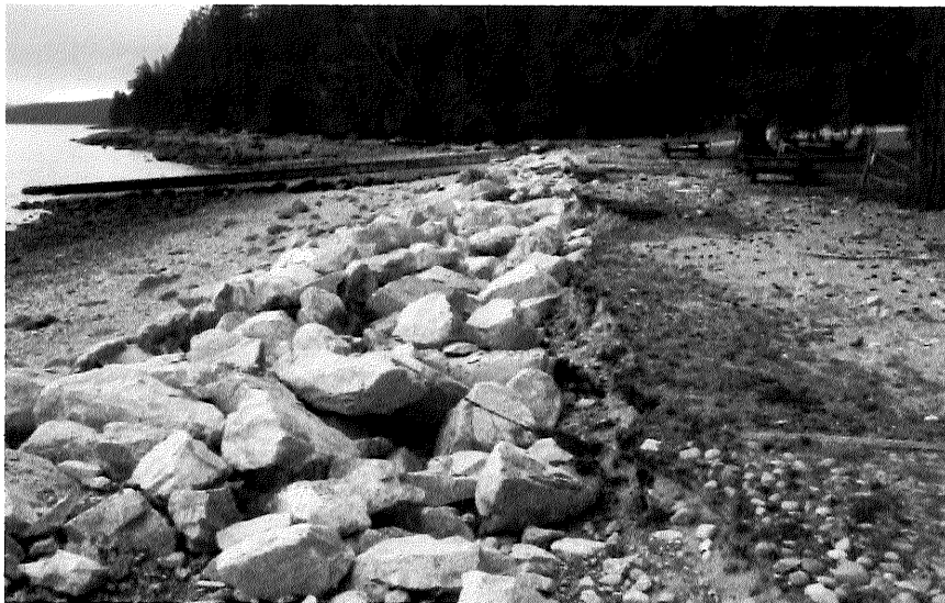
Rip Rap has been used to in the Park to curtail beach erosion
